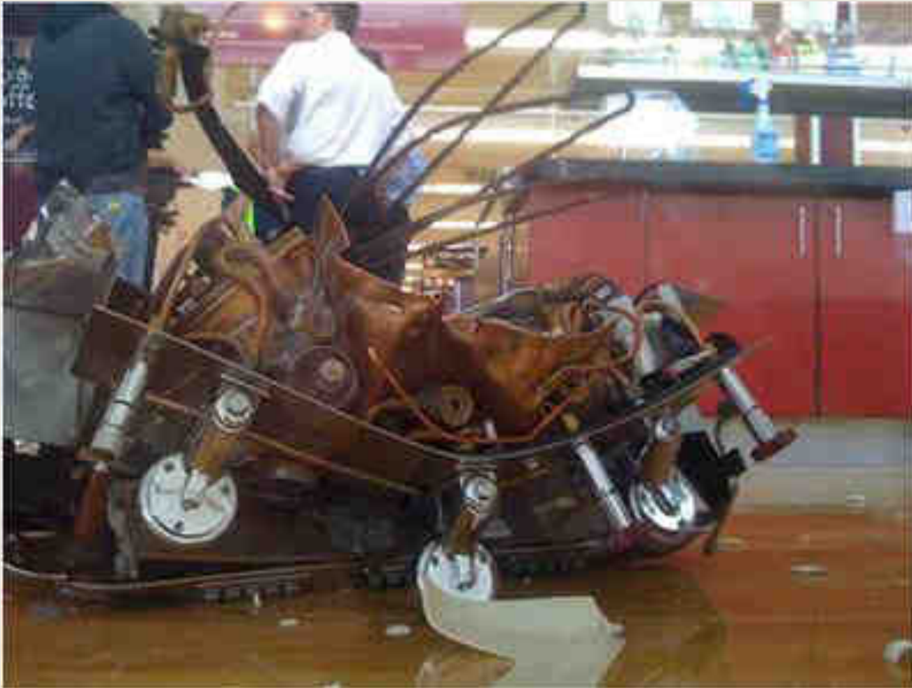
Failed Coffee Boiler
