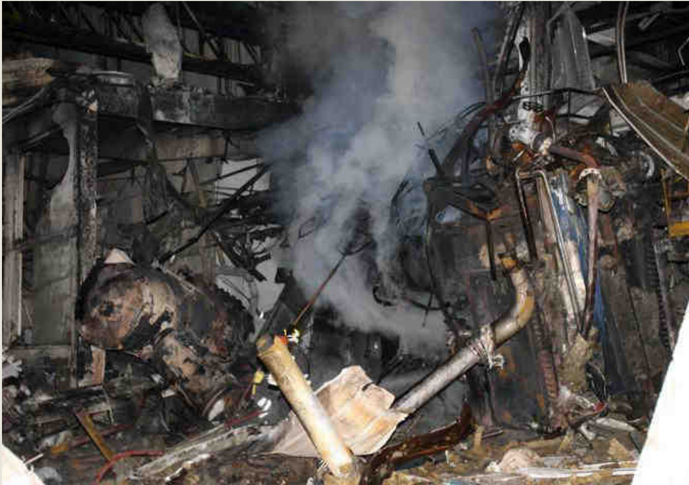
Failed Steam Boiler
