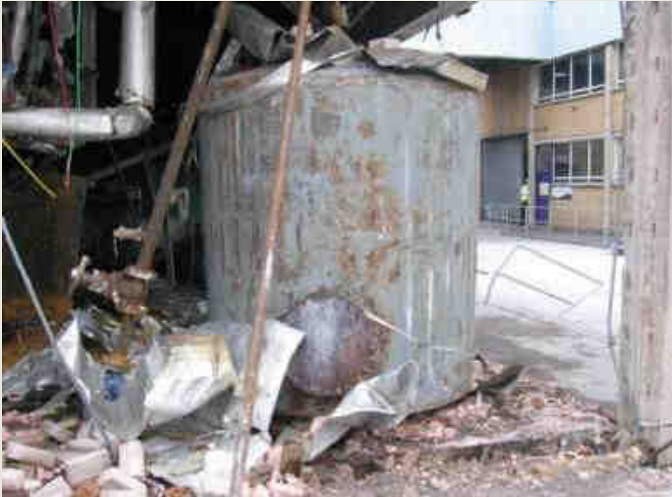
Failed Water Heater (Calorifier)
