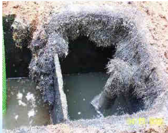
Collapse of Septic Tank due to lack of maintenance
